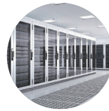
Large data center room
