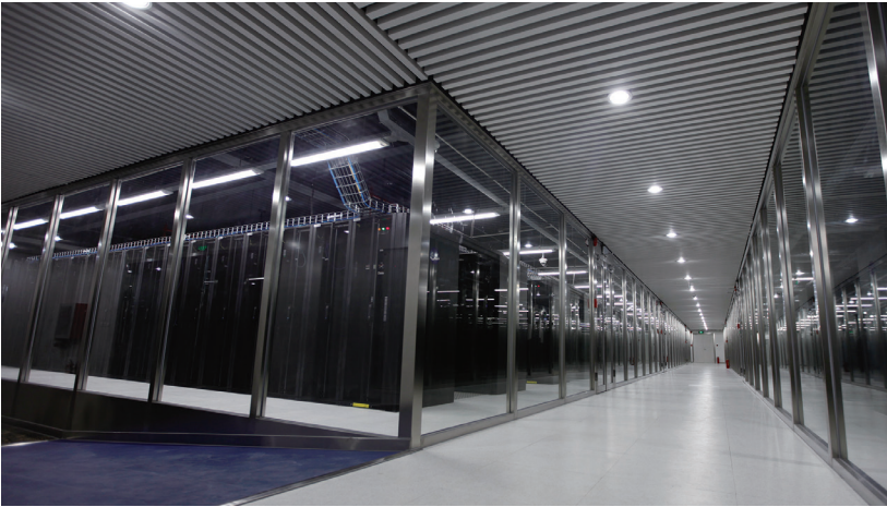
Beijing Kehua Zhongsheng Cloud Computing Data Center - Large Modular Data Center (the total construction area is 70,000 square meters)
