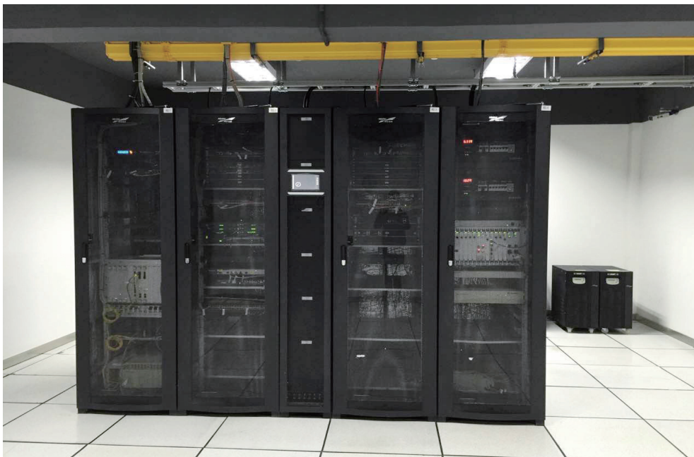
Gansu Construction Bank Information Construction - 1 set of Medium Modular Data Center
