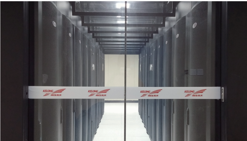
Guangdong Development Bank Chongqing Branch - Large Modular Data Center
